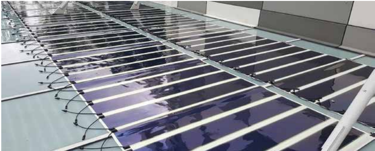
Fig. 6: Cleantech 2 building façade where HeliaFilm® has been installed on the roof and façade
