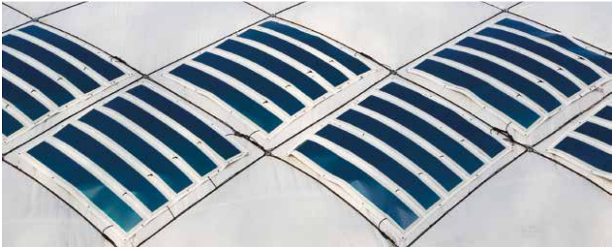
Fig. 4: HeliaFilm® on PVC – 1,5 kWp to support power needs for inflating the hall.:
